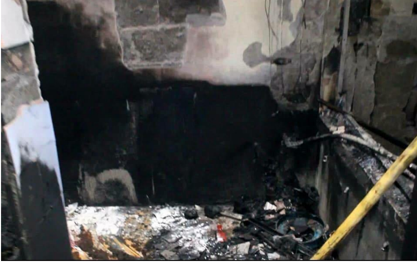
Figure (243) Damages caused by artillery and mortar shells fired by the Kurdish militia on the Turkmen houses in Altin Kopru, Kirkuk- TURKMENELI
