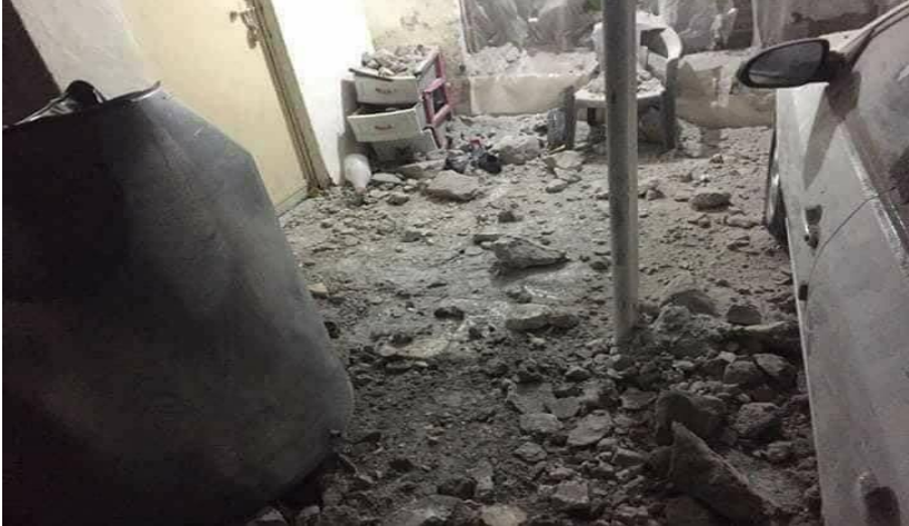
Figure (253) the damages on the Turkmen property caused by Kurdish militia firing Mortars shells in Tuz Khormatu
